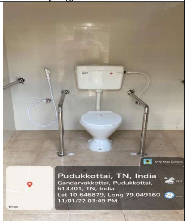
Divyangjan Toilet view IV
